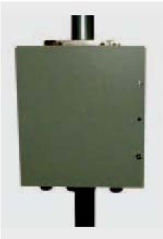
Figure 44 Pole mounted CMM3
