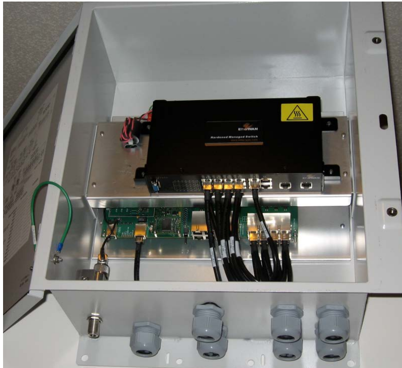
Figure 42 CMM4 (Cabinet with switch)
