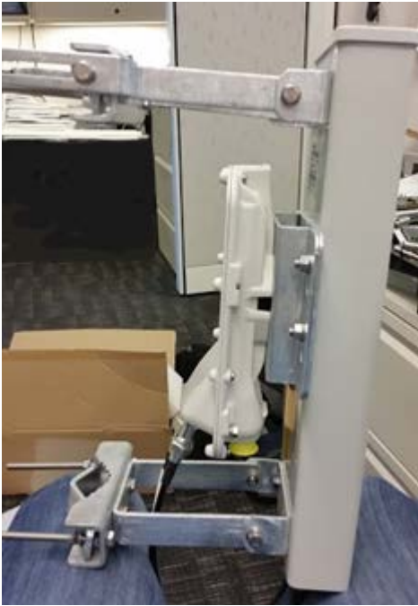
Figure 95 Completed AP and antenna assembly
