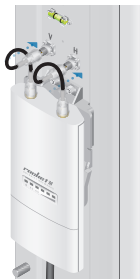
Connecting to a Sector Antenna
